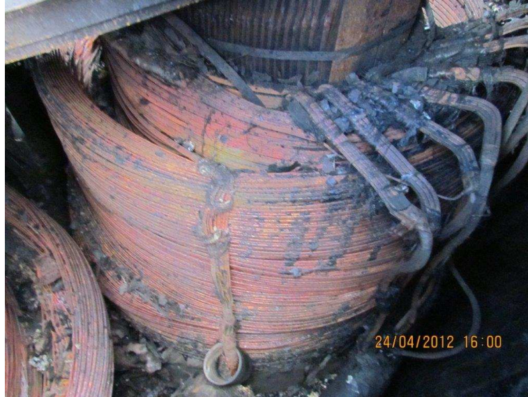
Figure 6. A damaged high-energy transformer
