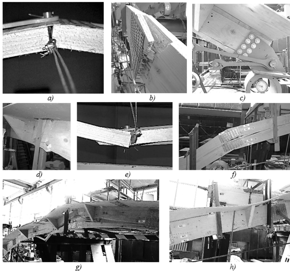
Fig. 10. The view of arches after being damaged: a) A-1.1; b) A-2.1; c) At-1.1; d) At-2.1; e) A-3.2; f) A-4.2; g) At-3.2; h) At-4.2.
