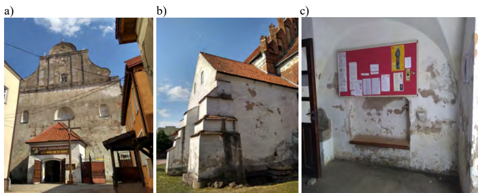
Fig. 1. St. Andrew's church in Barczewo - a) main entrance b) damaged side elevation c) multiple traces of damp visible on the walls from the inside
