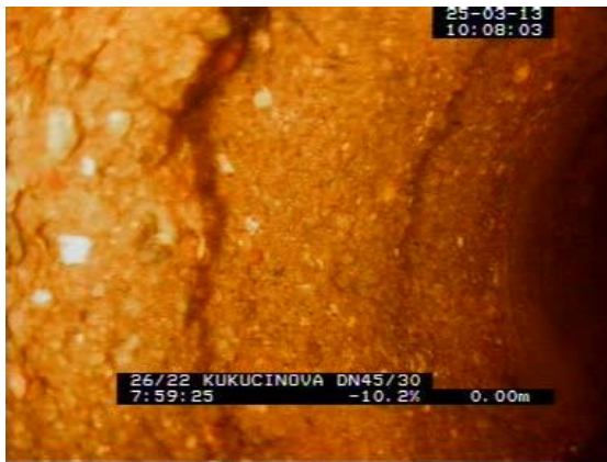
Fig. 3 Sewer pipe deteriorated by sulphate corrosion caused by microorganisms
