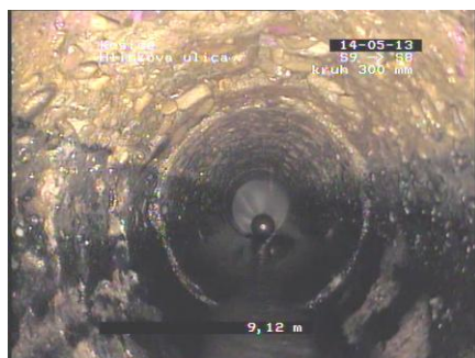
Fig. 4 Sewer pipe deteriorated by sulphate corrosion – cement matrix is disrupted
