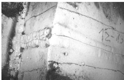
Fig. 3. Cracks of the bridge beam detected by the magnetic-powder method: a) type „Z1” joint 140 mm long; b) type „O” plate under the rail, 380 mm long
